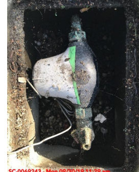
Meter on its Side
