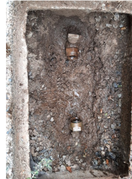
Meter Yoke Misaligned
